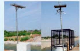
SCADA based automated system
